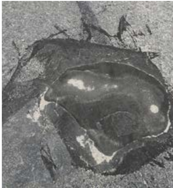
A photo of roadway requiring maintenance in Lake Los Angeles, submitted as part of the photovoice activity
